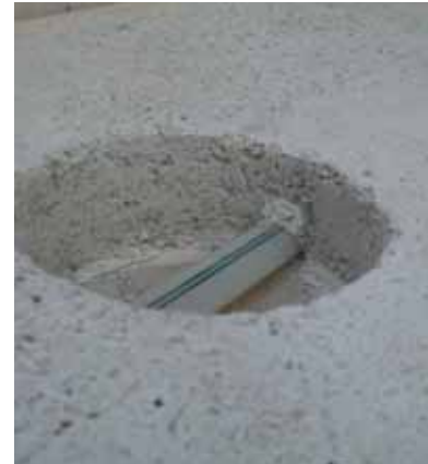
A heating pipe in the Glasscrete Screed.
